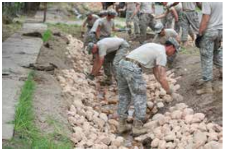
19th Special Forces Group (Airborne) Soldiers repair a run-off canal to help Spring City residents in Sanpete County.
