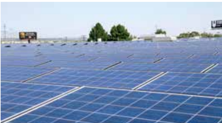
Solar panels on the Draper headquarters building.
