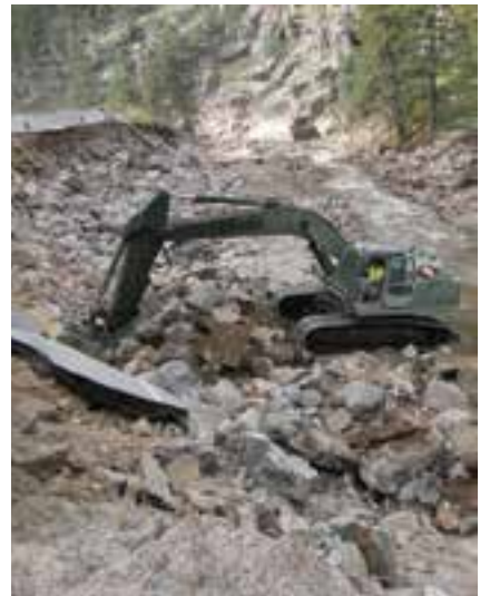
Units from the 1457th Engineer Battalion respond to Colorado flooding and the repair of Hwy 36.
