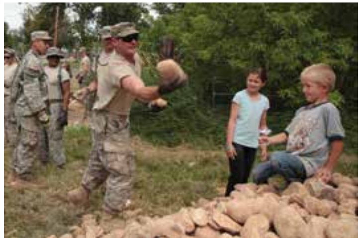
Members of the 19th Special Forces Group (Airborne) volunteered to help local Spring City residents repair a run-off canal during Operation skyline in Sanpete County.
