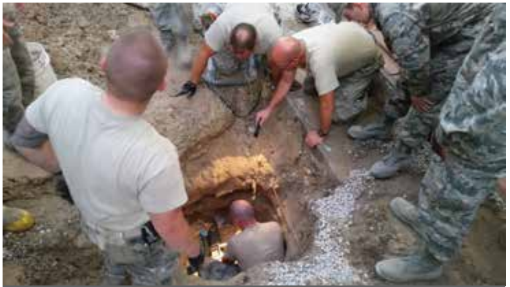
Senior Airman Loal Lee, 151st Civil Engineering Squadron, repairs a water leak at a deployed location in support of Operation Enduring Freedom August 26, 2014.
